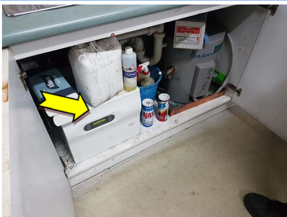
Photo 5. Interior, mezzanine level, kitchen, hot water heater – suspected SMF internal insulation material.
